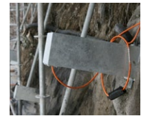
Rock anchor monitoring
