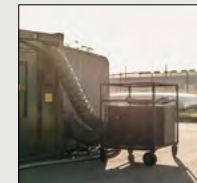
Militaryised HVAC unit with ducting
