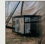
Split unit HVAC
