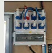
Internal power distribution
