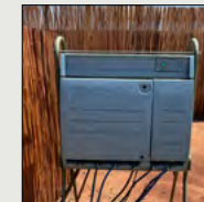
External power distribution
